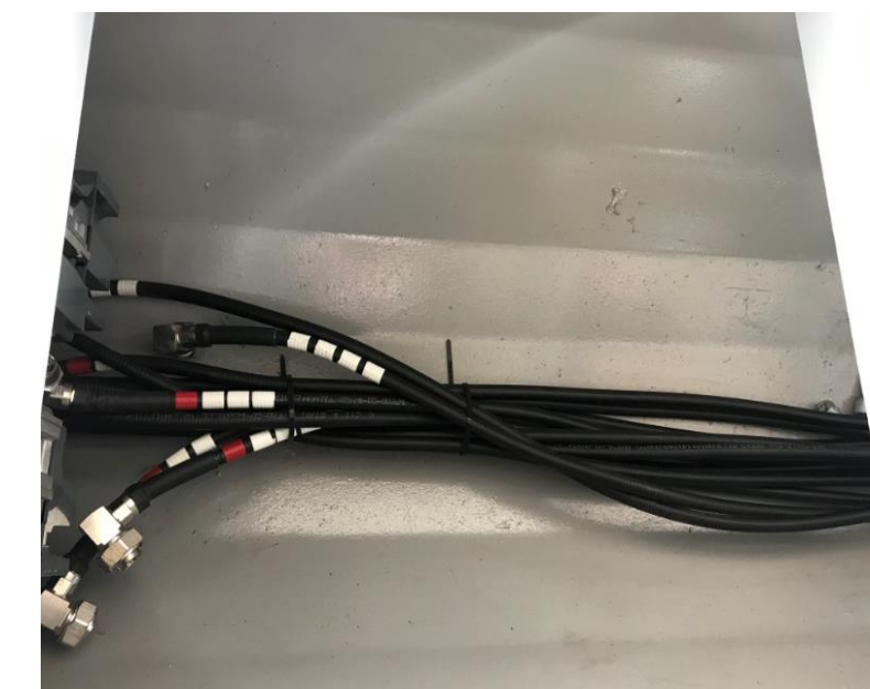
Cabos Fider 1/2" – Portas 3 e 4 (Outdoor)
